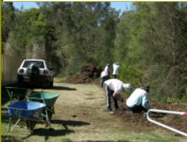
Green Team and Warners Bay volunteers mulching and planting in the Jones site riparian zone upstream of Jones Avenue in April 2008, after Hunter Water had laid the new sewer main. Funding for the repair of the site was provided by Hunter Water after negotiations with John Hughson, Landcare Co-ordinator.
